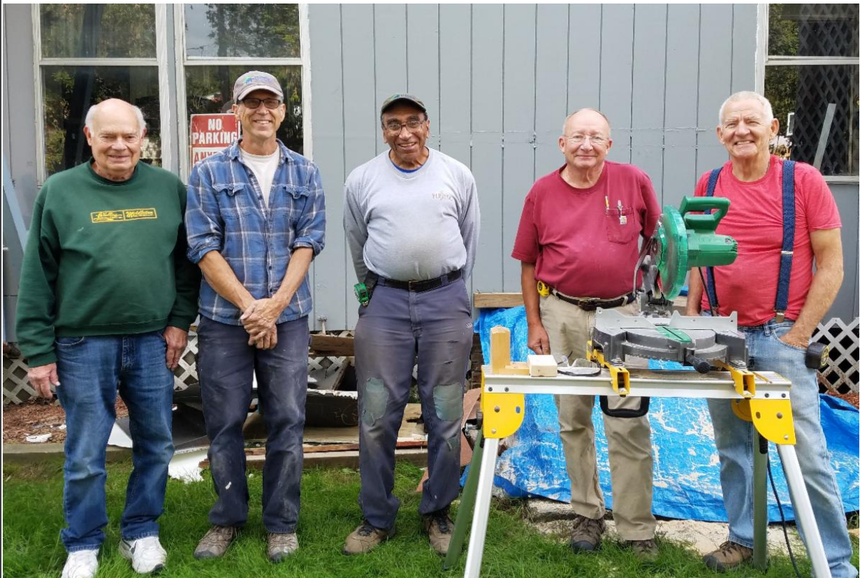
Gordon Best (veteran), PM John Heath, Charlie Clark (veteran), Dave Sherman, and George Imbrie take a break while renovating veteran Fran's bathroom.
