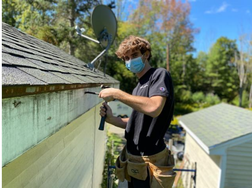
Volunteer Sam Lefkofsky removes fascia before moving onto building a stage & removing paneling.
