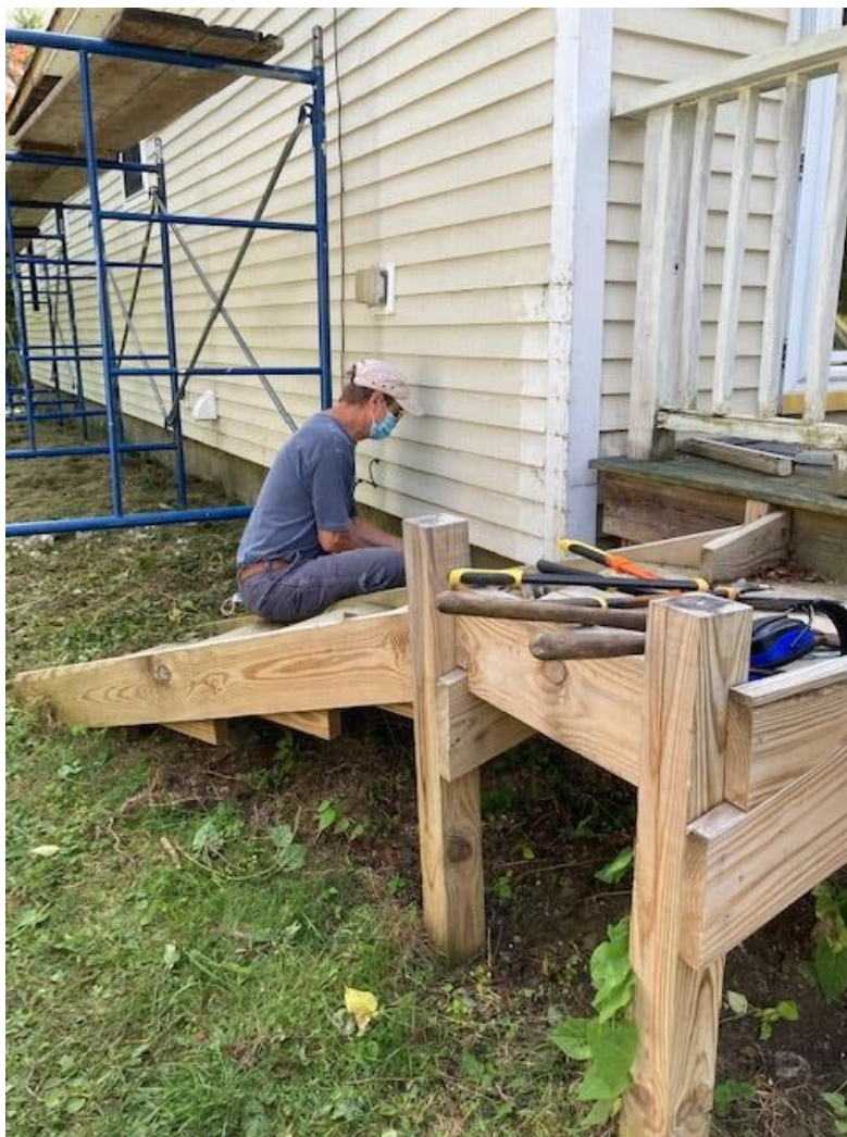
Board and Building Committee member Rick Biddle works on the north side of the home.
