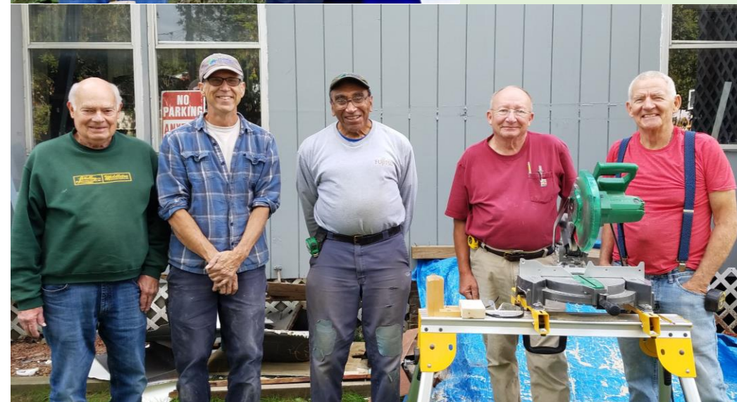
Veteran Gordon Best; UVHFH PM John Heath; Veteran Charlie Clark; Dave Sherman; & George Imbrie working on Fran's bathroom renovation this fall.
