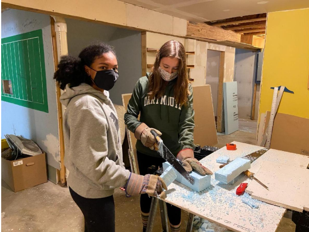
Dartmouth College Habitat Chapter volunteers work on an insulation project in the basement in October.
